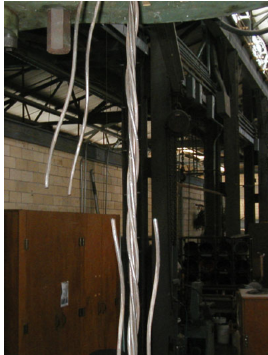
(b) Failure of CUT 3
