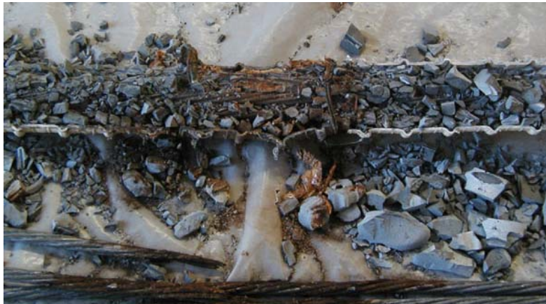
Figure 5.36 Condition of Grout in Vicinity of Void 1 after Autopsy
