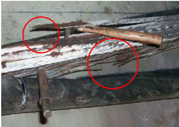
(a) Fractured Wires
