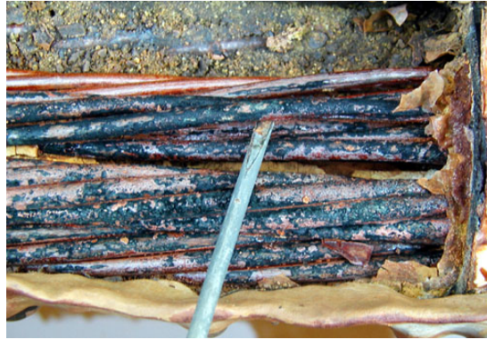
Figure 5.32 Observed Wire Breaks at Void 3 at Conclusion of Exposure Test
