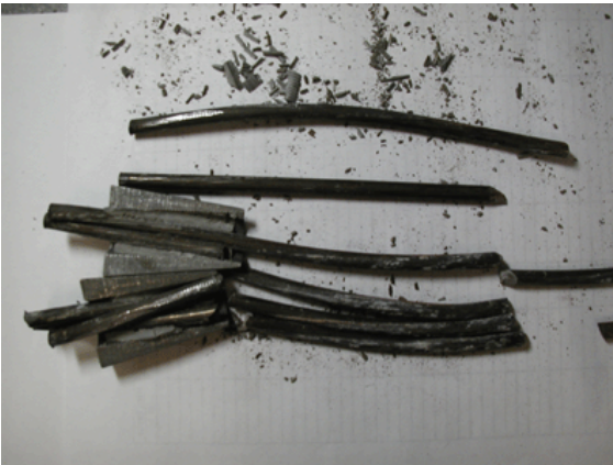
(c) Inside of anchor head (Bottom strand)
