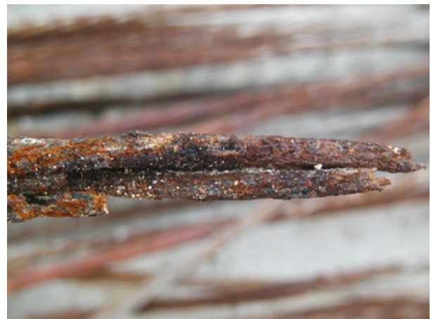
(b) Completely fractured strand
